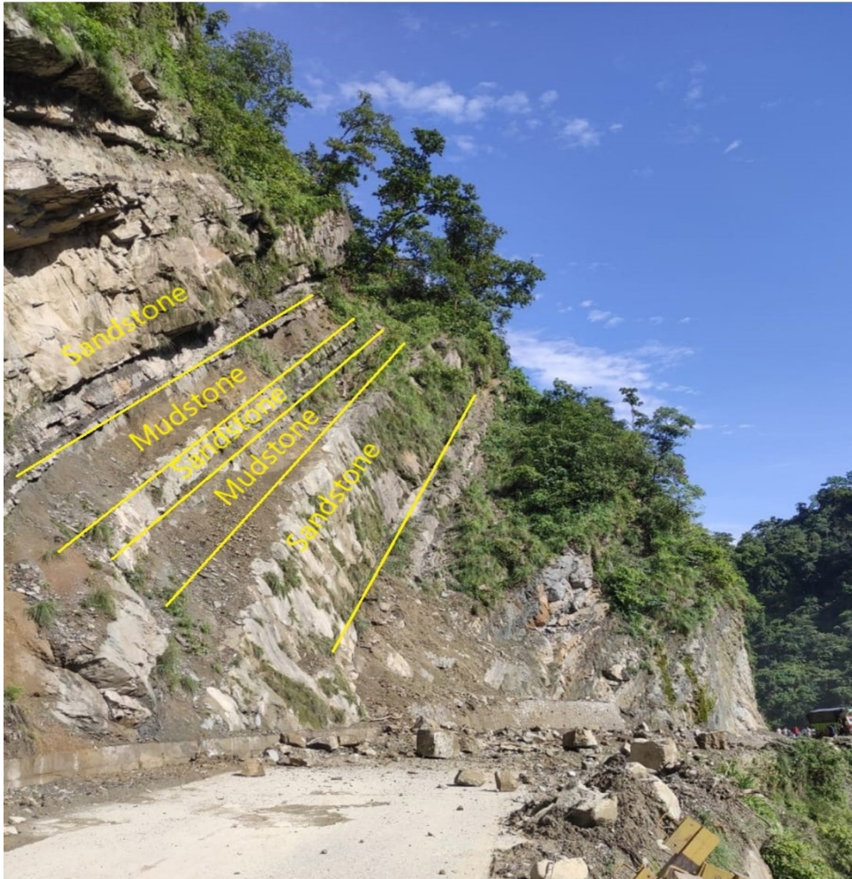
Figure 6: Alternating bands of sandstone and mudstone along with rockfall observed at the section of Siddhartha highway near Siddhababa Temple (GPS: 27°43'58.82" and 83°28'5.22")
