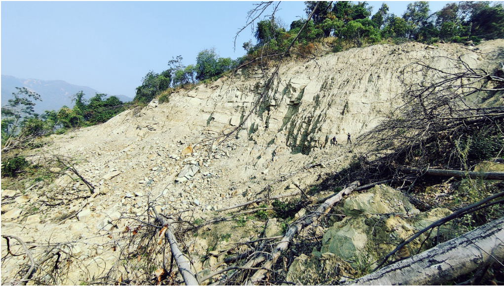
Figure 4: Crown of Shrawan Danda Landslide (GPS: 27°42'55.77" and 83°28'31.30")
