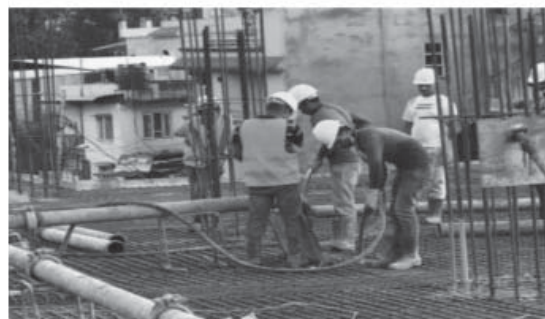
Figure 1 Hazards at Building Construction
