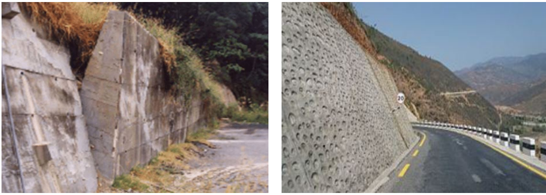
FIGURE 1. Left: Concrete retaining wall turned outward by slope failure above it during the Chi-Chi earthquake in Taiwan (1999). Right: Retaining walls constructed in the BP highway in the eastern Nepal where various slope stabilization techniques are adopted (Photo: N. Sitar).
