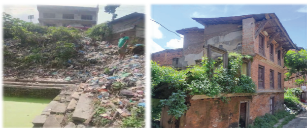
Fig 3 : Decaying of traditional Materials (on the left) Pukhus site used as dumping area (on the right)
