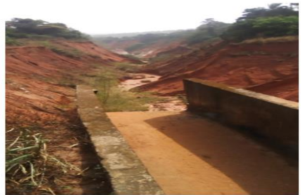
Plate 2: A concrete work of drain torn by the excess flood water entering the Abia gully, Udi Local Government Area, Enugu State, wreaking havoc on agricultural lands and water bodies
