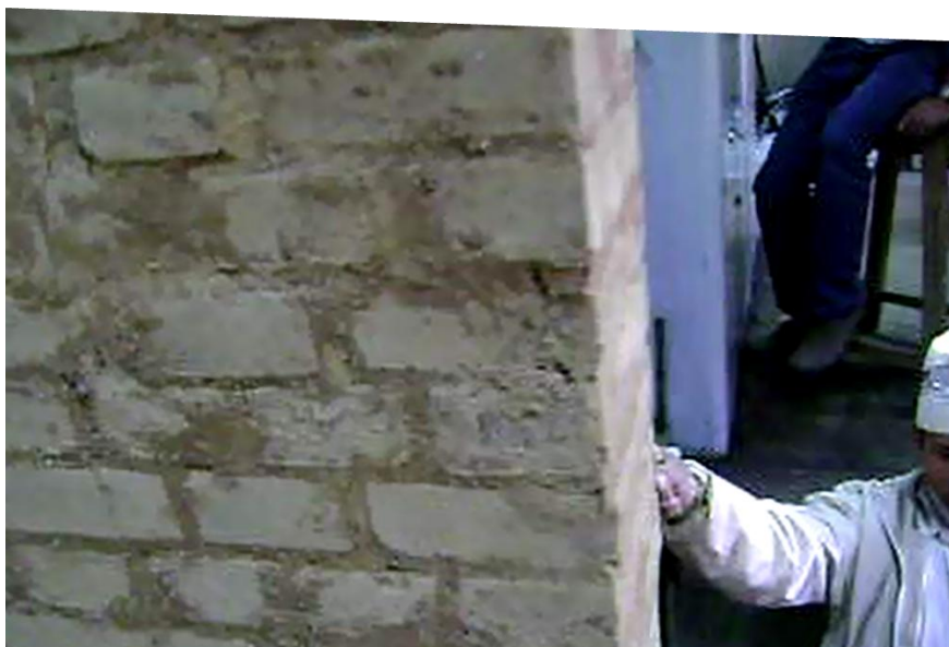
Figure 4: Cracking of CSEB masonry wall for a monotonic compression load (Bhatt., 2015)
