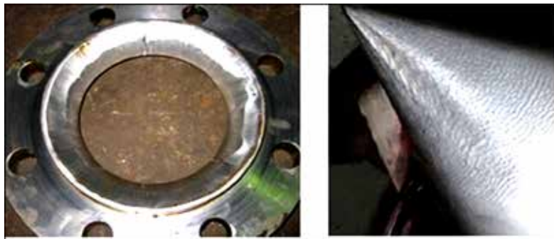
Figure 4: Erosion in nozzle and needle (On left, erosion in nozzle ring of Andhi Khole HPP, Nepal and needle erosion in Khimti HPP, Nepal (Adapted from Neopane et al. 2011))
