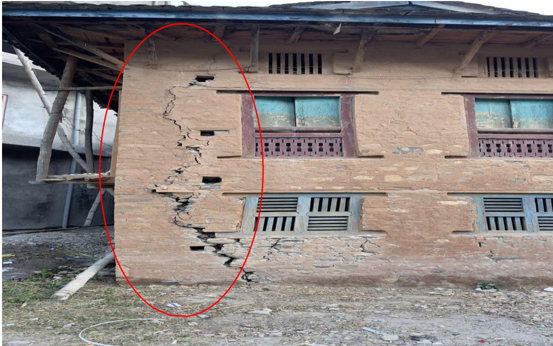
Figure 10: Severe Cracking due to Inadequate Lintel Beam.
