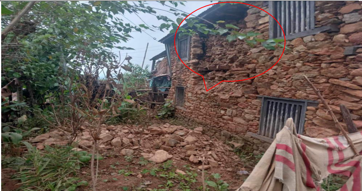
Figure 8: Delamination of the exterior walls
