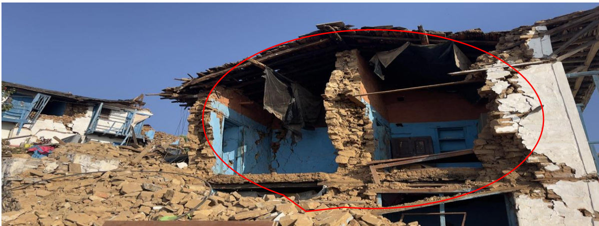
Figure 11: Out of plane failure of exterior walls
