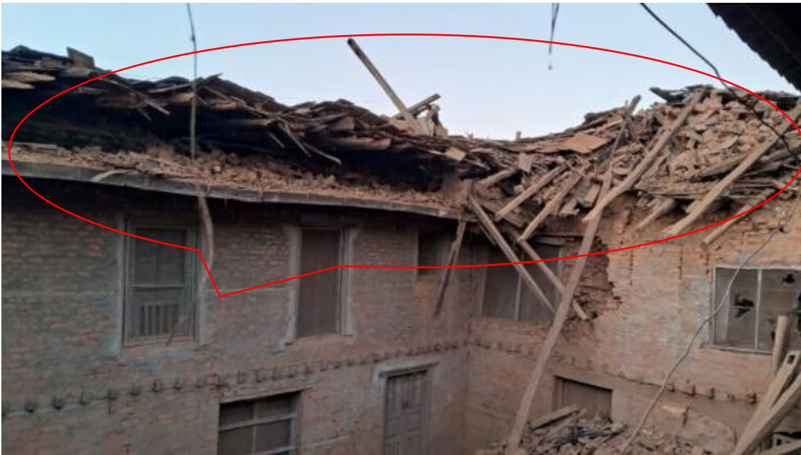
Figure 9: Complete Collapse of Roof and Gable wall
