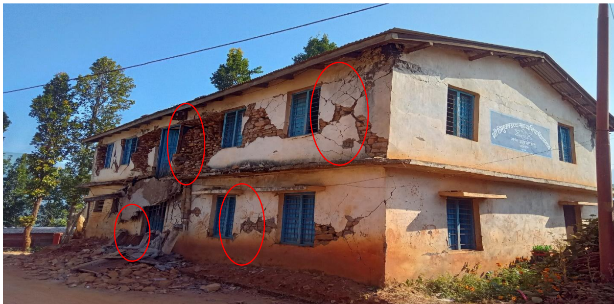
Figure 17: Failure due to excessive number of openings
