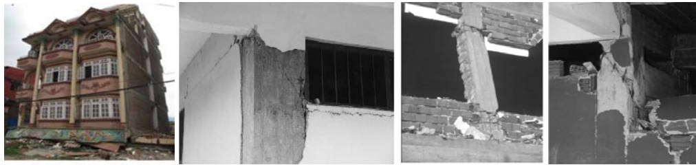
Figure 3: (a) Soft story failure; (b) Short column effect due to window opening; (c) and (d) Short column effect due to partial height of masonry infill wall [8]
