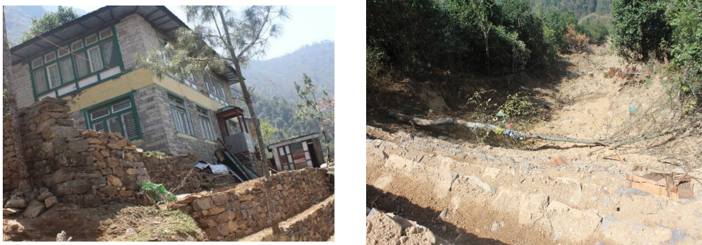
Figure 5: Wall constructions to mitigate house and trail at Surke village a) landslide affected house upper part b) wall construction (stone and mud) to control headward extension of landslide.
