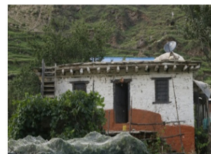
Photo 4.3: Stone Masonry Building with improvised Door and Windows (Shahi, Saroj 2022)
