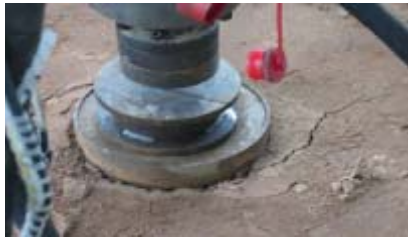
Fig. 5. Cracks at the sub base surface
