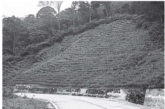
Figure 11: Steep batter stabilized with vetiver – Ho Chi Minh Highway, Vietnam
