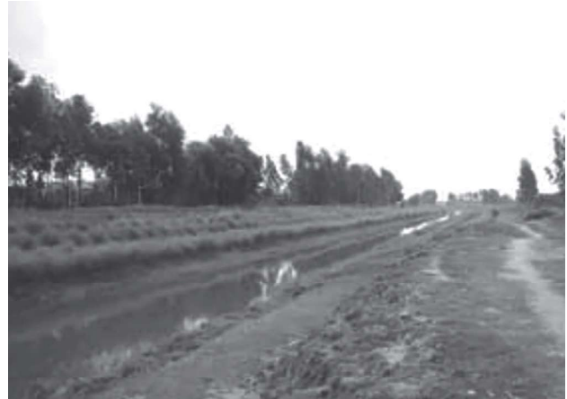
Figure 6: a section of the irrigation canal, surface erosion mars the opposite bank
