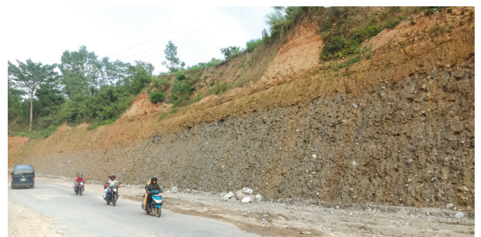
Fig. 3: Cut-slope excavated on debris material along the roadside at Yampa village, Prithvi Highway.
