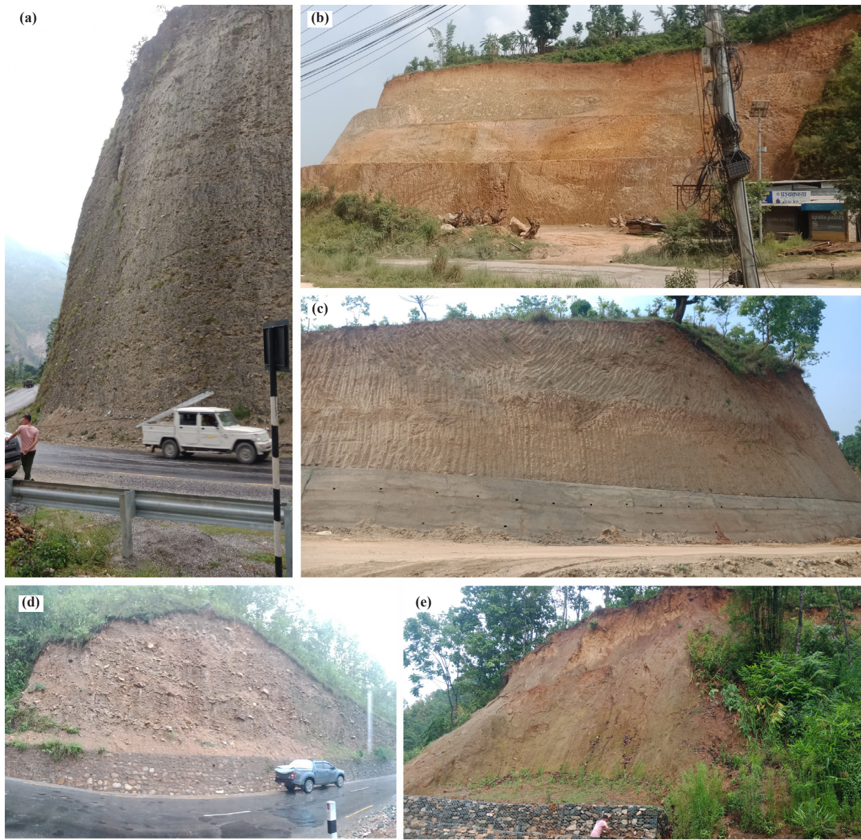
Fig. 6: Cut slope at road section from central and western Nepal (a) conglomerate at Maldhunga–Kushma road, (b) slope with benching on residual soil at Dumre Bazar, Tanahun, (c) residual soil at Bhansar, Tanahun, (d) near Kushma Bazar, (e) red soil cut slope at Kushma–Dimuwa section.
