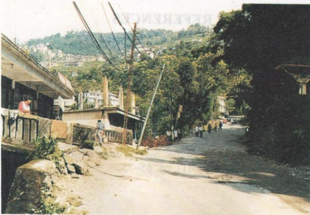
Plate 3: The sinking part of the National Highway 31A at “Six Miles” Landslide, Tadong
