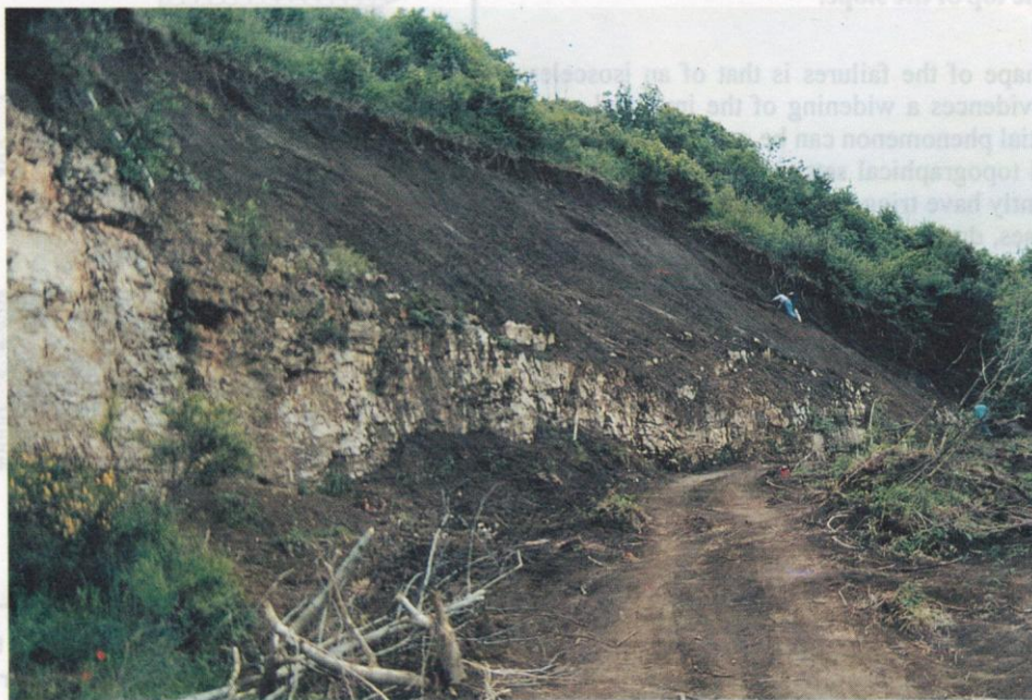
Plate 4: Typical failure above a track
