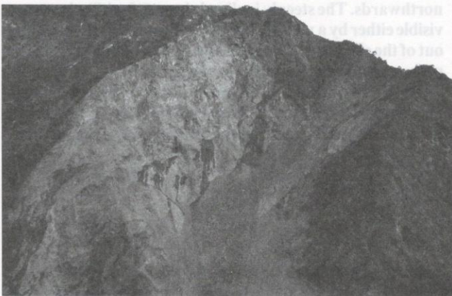
Plate 10: This picture shows some features of Plates 8 and 9 in more detail, especially the potential failure sites adjacent to the recent one. Also note the faulted left part of the frontal mountain pyramid with its precipice, namely a relict failure scar at the Kali Gandaki Valley slope in the foreground.
