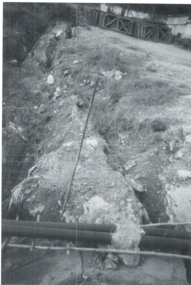
Fig. 3: Riverbank cutting and block fall by the side of Seti River at highway bridge site.
