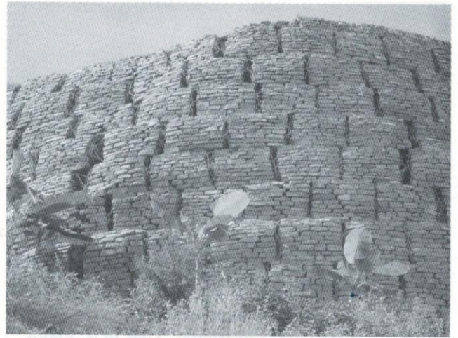
Fig. 14: Open joints between the gabion boxes of Loop No. 8. View to SW. Photo by M R Dhital.
