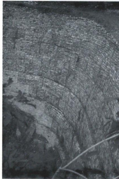
Fig. 9: The gabion wall is bulging near its base at DJ32. View to SW. Photo by Cris Grant.
