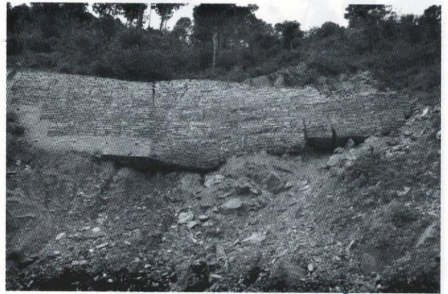
Fig. 8: Partly damaged gabion wall and overhanging stone masonry wall at DJ31. View to W. Photo by Cris Grant.
