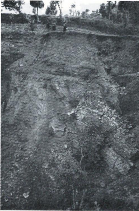
Fig. 6: Damaged road and failed gabion walls in the Narsinge Khola northeast of Halesi. View to NE. Photo by Cris Grant.
