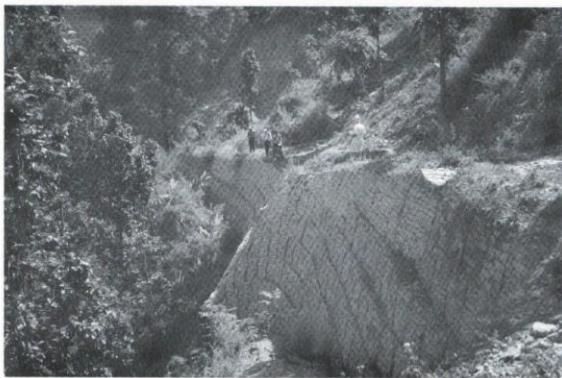
Fig. 16: Partly damaged and bulging wall east of Loop No. 6. View to NE. Photo by Cris Grant.
