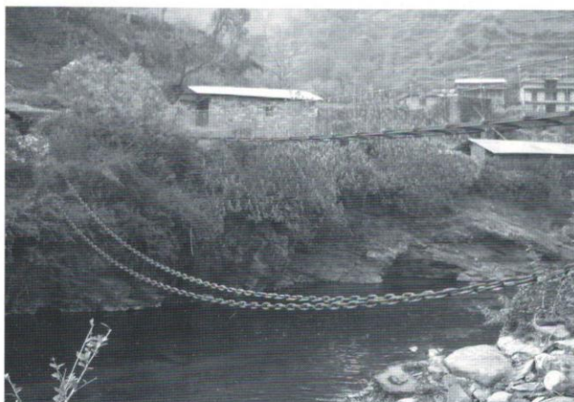
Fig. 5: Iron chain (Sikri) made up of Thoshe iron used in suspension bridge (lower level) over Khimti River
