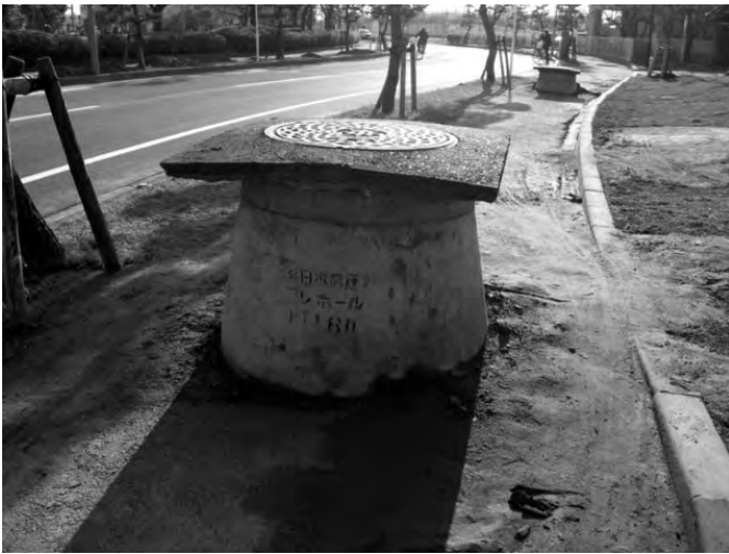
Fig. 1: Manhole uplifted during earthquake March 2011 in Urayasu area.
