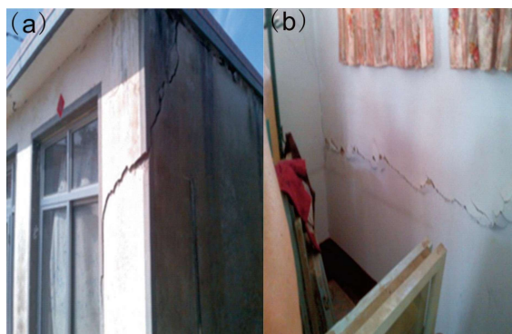
Fig. 4: Damage of buildings. (a) tension failure and (b) shearing failure
