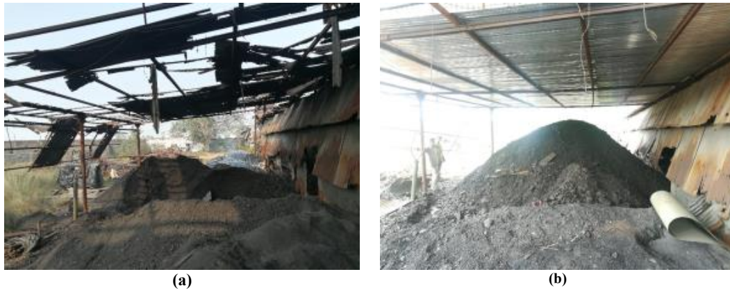
Figure 7: (a) Before: damaged roof of coal storage shed (b) After: coal stored under the repaired roof
