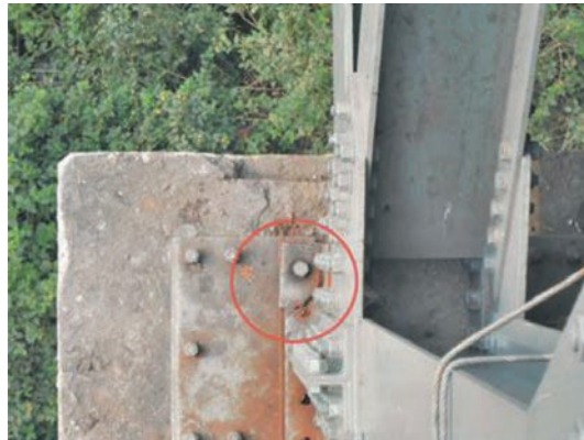
Fig. 1: Failure of the bolts in the gusset plate near to the left end
