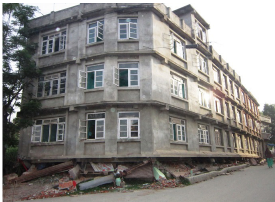
Figure 3. Soft-first storey failure of 4 storey building in Chamati, Kathmandu
