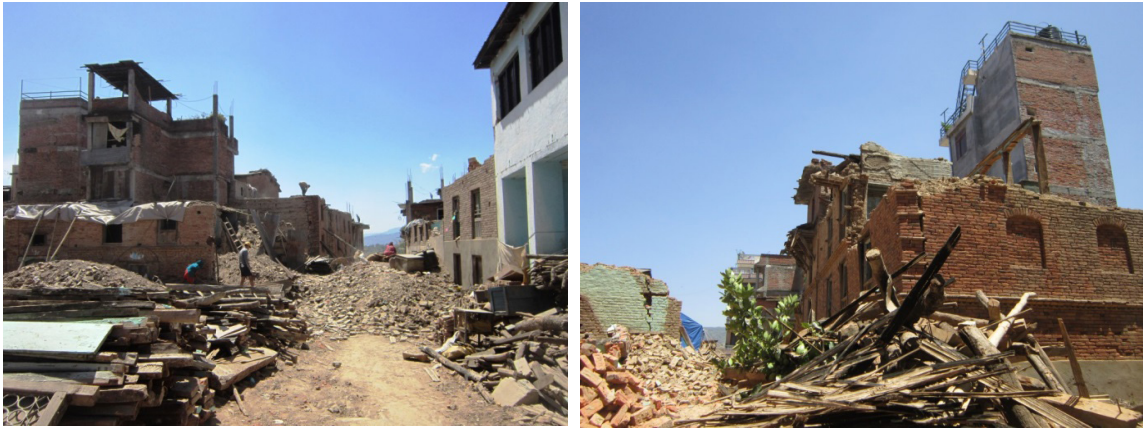
Figure 5. Collapse of old brick masonry buildings and still standing RCC building in Sankhu, Kathmandu.
