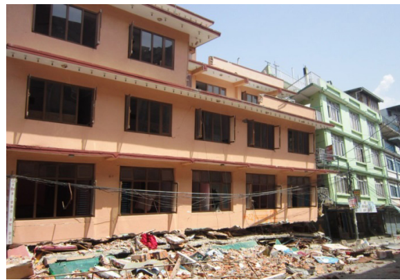
Figure 4. Soft storey failure of a guest house building in Gongabu, Kathmandu
