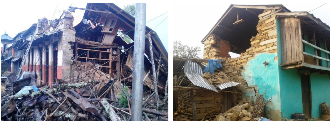
Figure 6. Collapse of stone masonry buildings with mud mortar Pipalhok village, Gorkha
