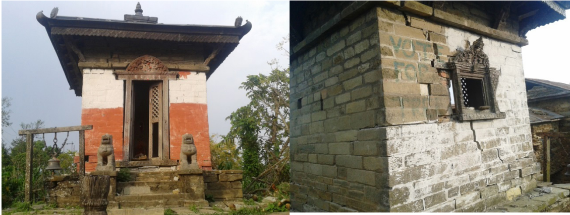
Figure 7: Diagonal Shear cracks at two side faces of Vimsen Temple at Phinam-5, Gorkha
