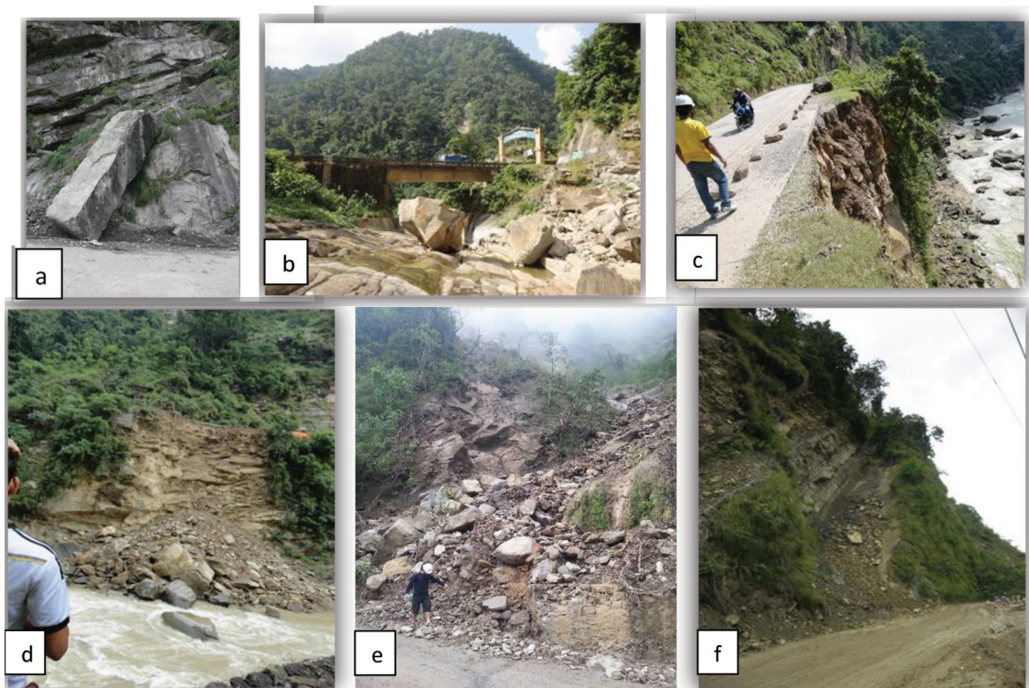
Fig. 5. Rock slope failure problem (a, b), Block failure type (c, d), Slope scar collapse and Debris flow (e & f).
