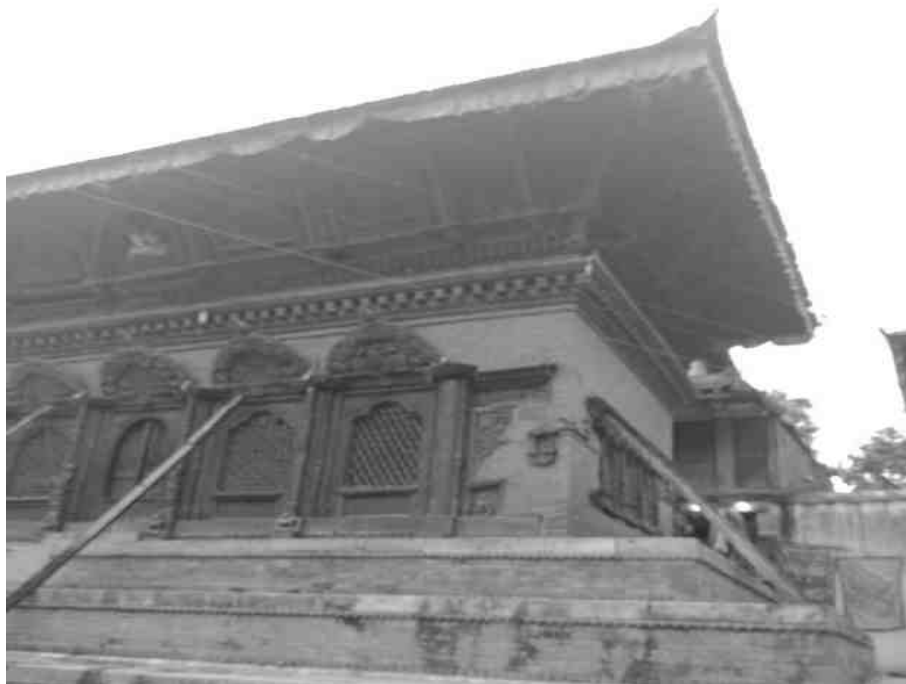
Figure 18: Failure of masonry structure of Shiva Parvati temple
