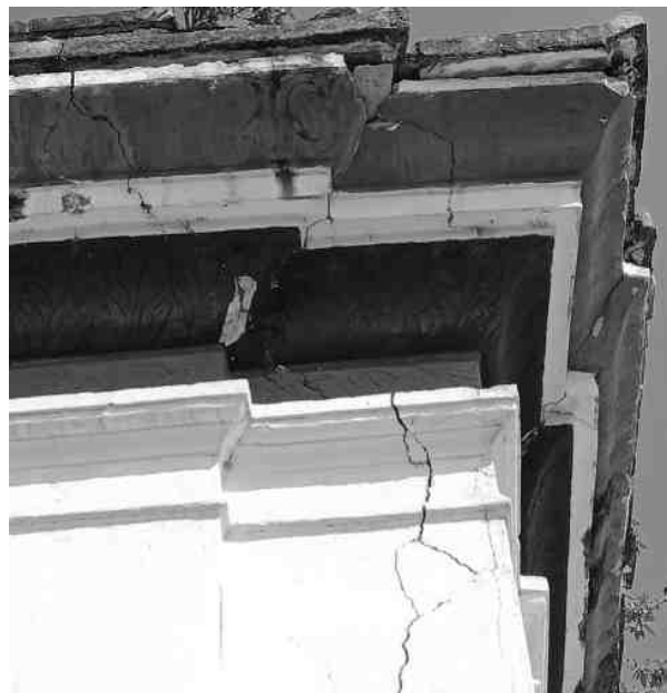
Figure 24: Crack near the roof of Narayan temple in Kalmochan (Photo source: Author)
