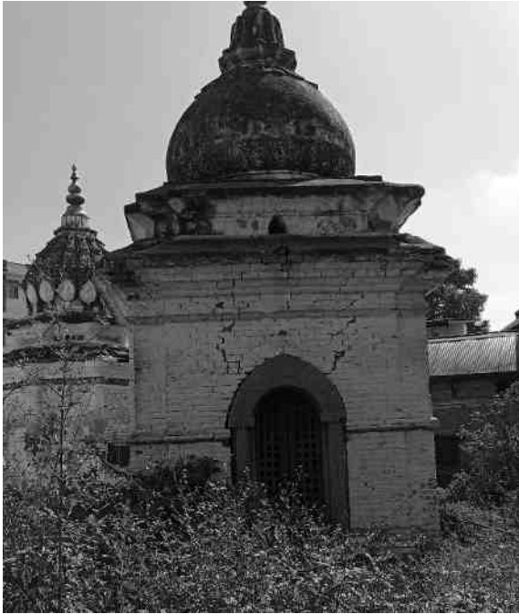
Figure 25: Crack over opening in brick masonry in Mahadev temple of Kalmochan premises
