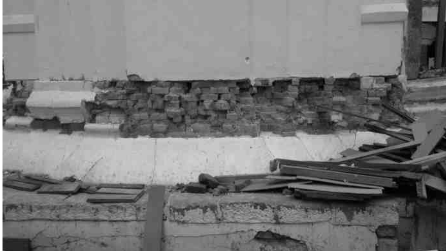
Figure 17: Collapse of Anantapur temple in Swayambhu premises, Kathmandu (Photo source: author)
