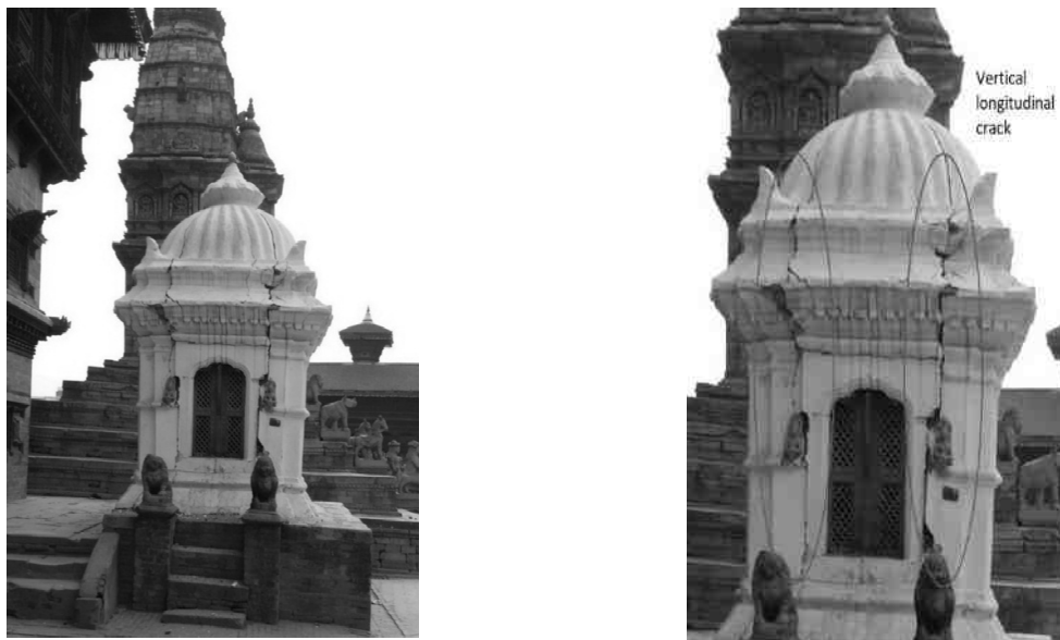
Figure 3: Longitudinal vertical joint failure of Shankernarayan Temple of Bhaktapur Durbar Square (Photo source: author)
