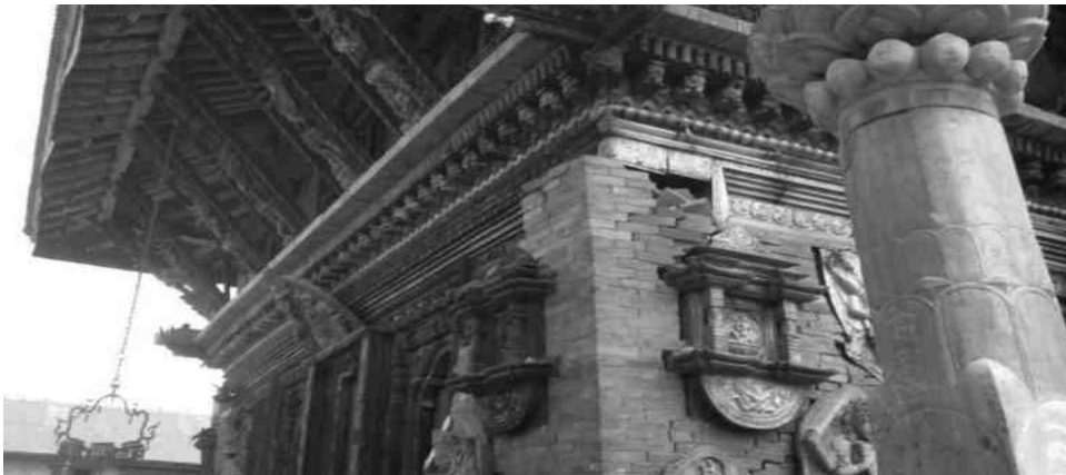
Figure 10: Damage in Changu Narayan Temple (North-West corner, top)
