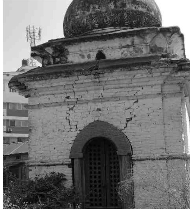
Figure 26: Close view of crack over opening in brick masonry in Mahadev temple of Kalmochan premises
