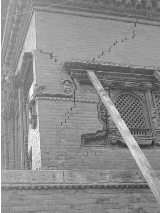
Figure 19: Diagonal shear crack in south east corner of short side elevation (Photo source: author)
