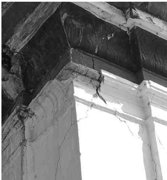
Figure 23: Crack near the roof of Narayan temple in Kalmochan (Photo source: Author)
