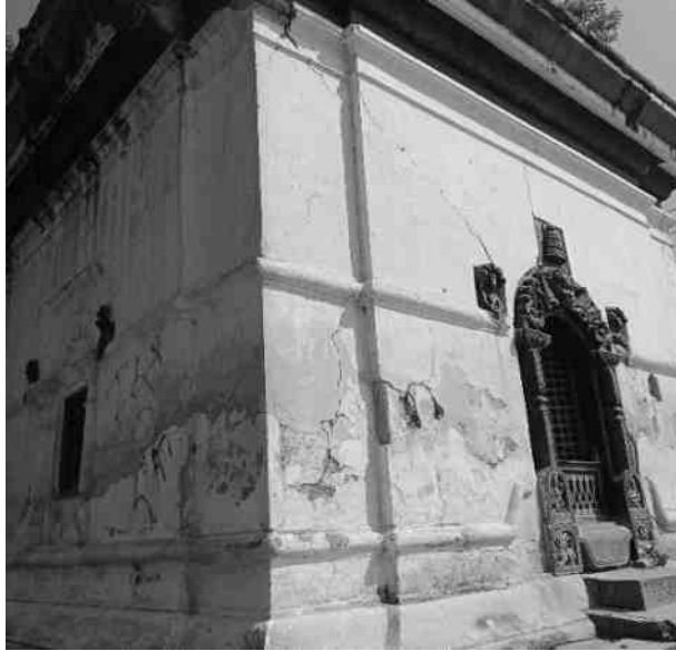
Figure 21: Wall crack in Narayan temple of Kalmochan (Photo source: author)
