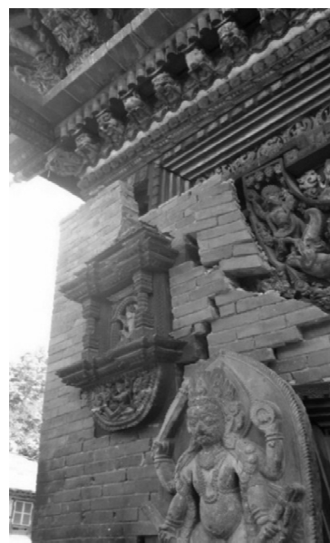
Figure 12: Damage in Changu Narayan Temple (North-East corner)
