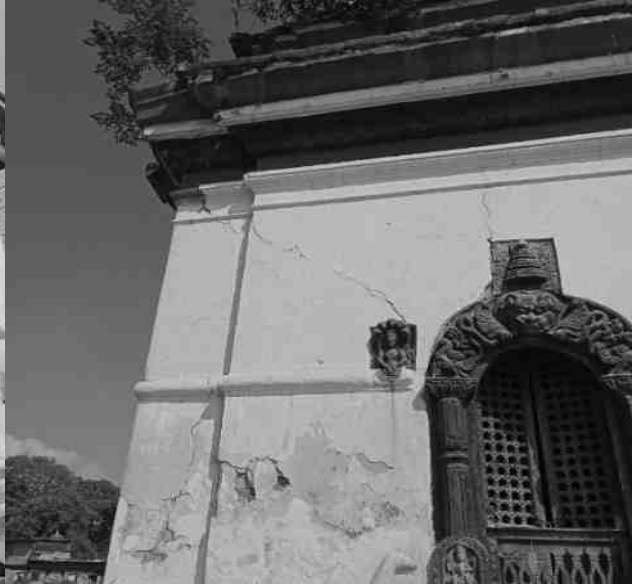
Figure 22: Wall crack in Narayan temple of Kalmochan (Photo source: author)
