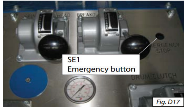
Figure 11: Emergency stop button for the operation
