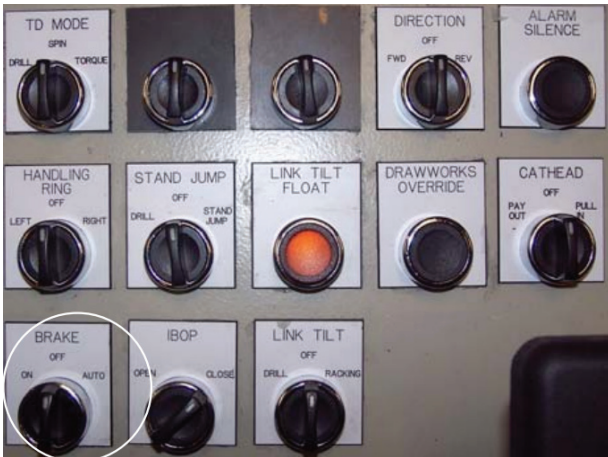
Figure 2: Top Drive control panel in drillers console
