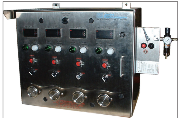
Figure 12: Mud pump control center
