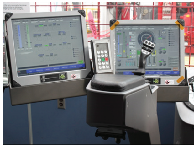
Figure 13: Joystick (TD control) and HMI at the drillers cabin
