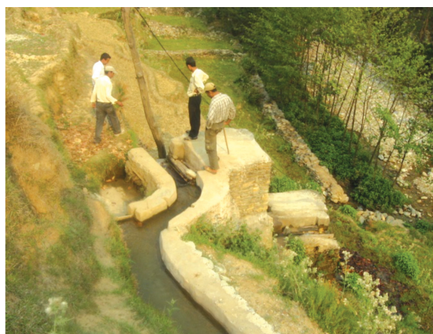
Figure 2. Two Pico-Hydro Low head Turbines in Series, Gulmi.
