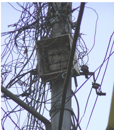
An overburden Distribution Line
