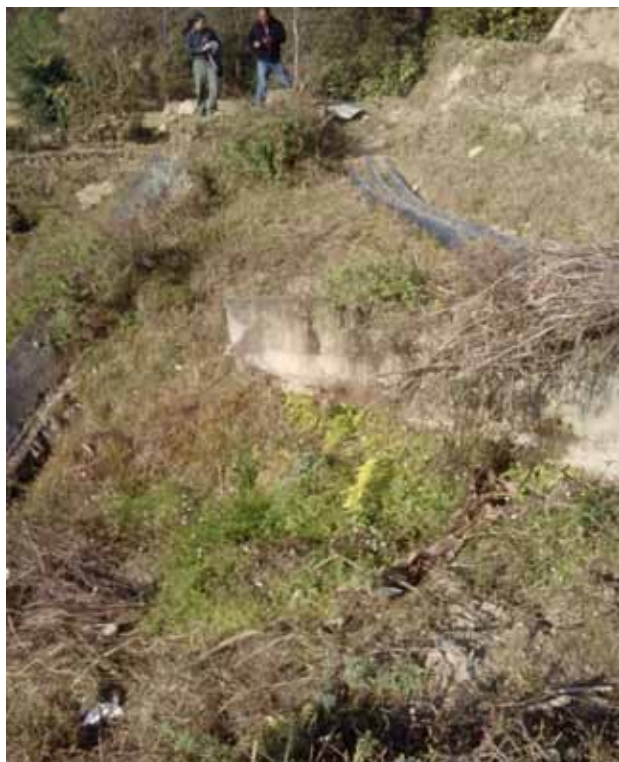
Photo 6: HDP Pipe used as emergency material at RCC canal breached section
