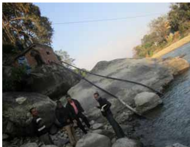
Photo 7: HDP pipe used for lift irrigation
