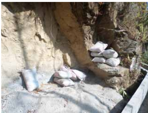
Photo 3: Cement storage at site: example of improper storage
