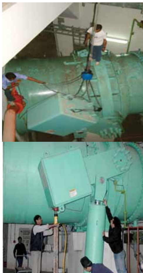
Photo 2: Photos of opening of inlet valve by using 3 ton chain block and 20 ton hydraulic press.
