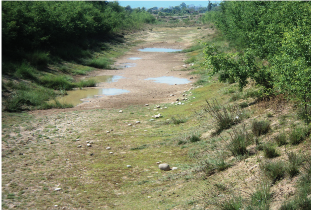
Photo 1: A part of the already dug 3 Km Nepal canal from the Tanakpur barrage at EL. 241.25 meters in the Nepalese territory (courtesy Mr. R. R. Lumsali)
