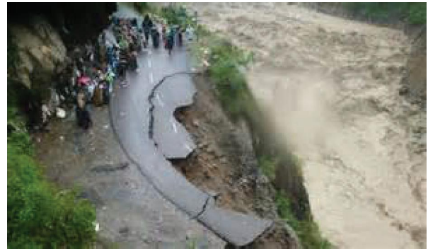
Figure 9. Road to Gaurikund collapsed
