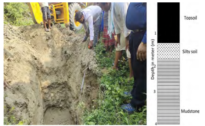
Fig. 10: Excavation of pit P2 (left) and lithology (right) at Samari Bhanjyang (GPS: 27.122785N, 85.597321E).
