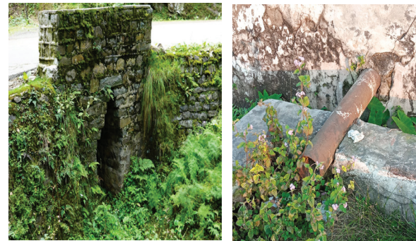
Figure 7: Abandoned dried-up spring (left) and dried water boring (right) in Shuklaphanta municipality-8
